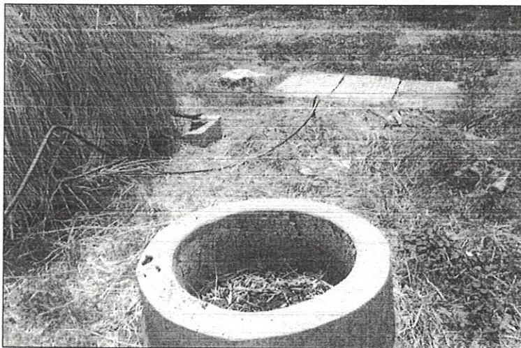
Plate 6 Improper alignment of gas pipe in Mandya
