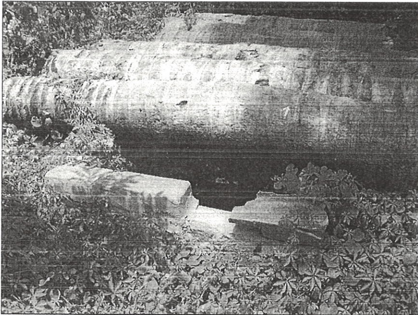
Plate 10 Damaged outlet tank without a proper cover in Uttara Kannda
